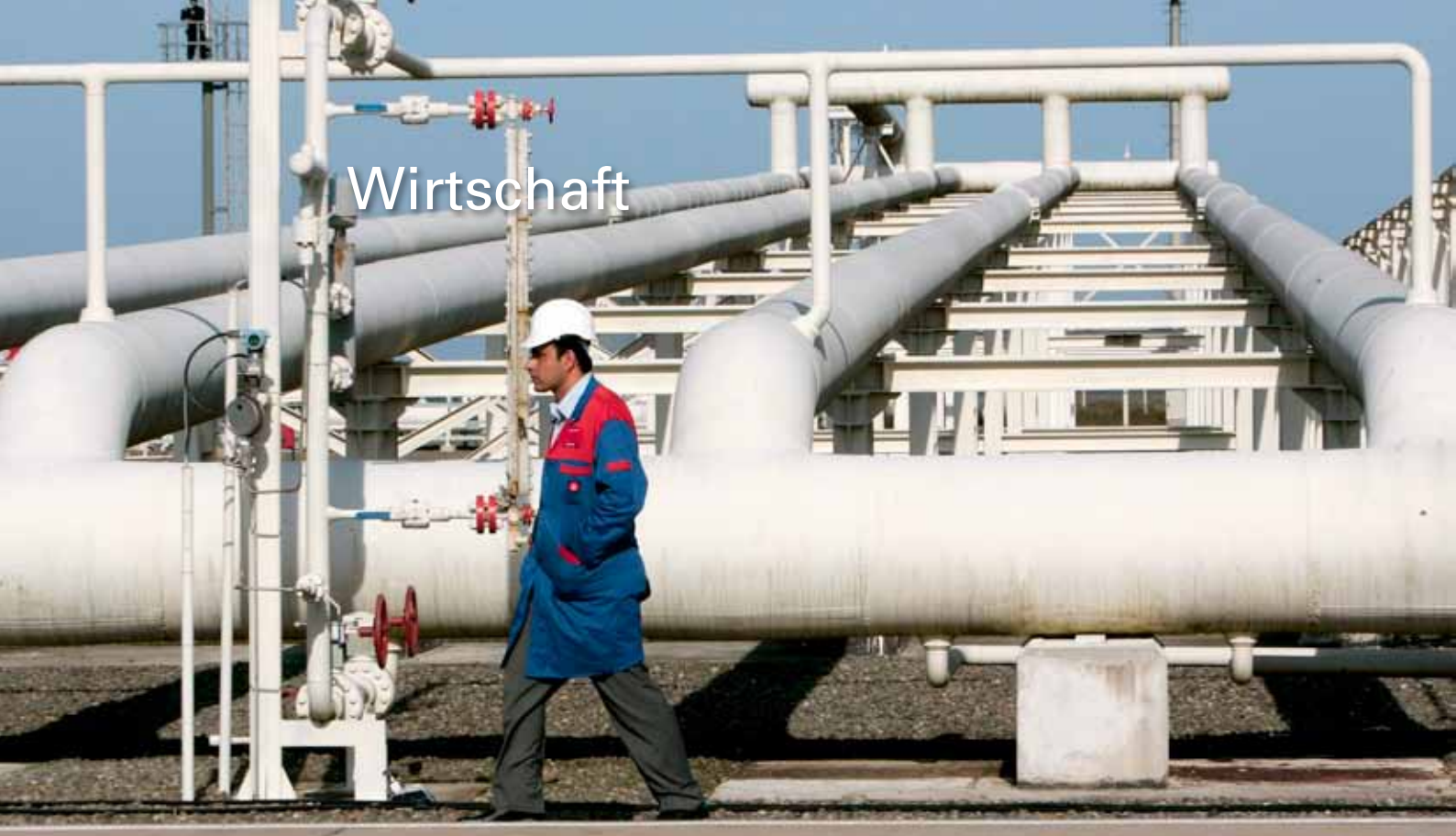
Durusu in Northern Turkey: The gas pipeline "Blue Stream" carries natural gas through the Black Sea from Russia into Turkey
